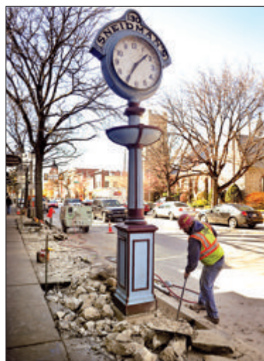
Press Enterprise/Bill Hughes MATTHEW SNYDER , Wolyniec Construction of Williamsport, breaks up blocks of sidewalk along East Main Street in Bloomsburg on Monday. The project will replace the old cobra-head street lights and blocks of sidewalk close to the curb.
